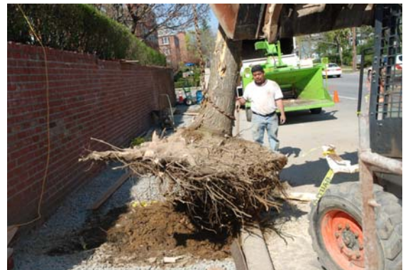
TREE STUMP REMOVED FROM SIDEWALK
